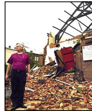
Bishop Johnson observes the tornado damage of 05/04/03
